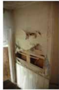
broken lath and plaster
