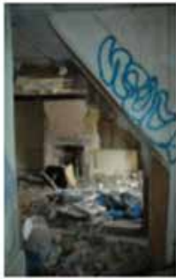
trashed partition wall to corridor
